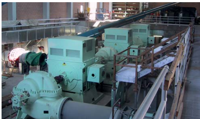
Customer: San Diego County Water Authority Country: USA
