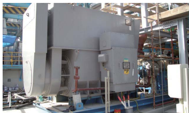
Customer: Jebel Ali Power and Desalination Station Country: Dubai
