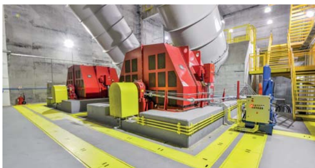
Customer: CPFL - SHP Salto Goes | Country: Brazil
