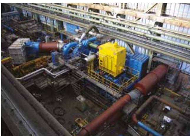
Supply: 14,000 kW, 10,000 V, 4 poles, frame 1000 Application: Test laboratory
