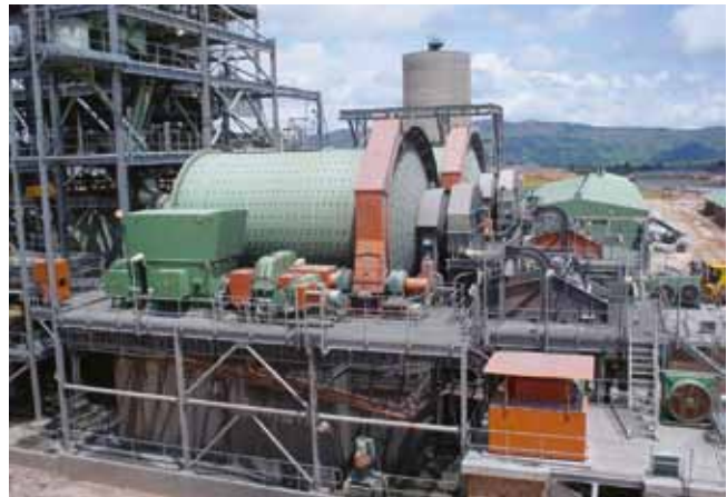
Supply: 6,500 kW, 11,000 V, 6 poles, frame 900 Application: Ball mill
